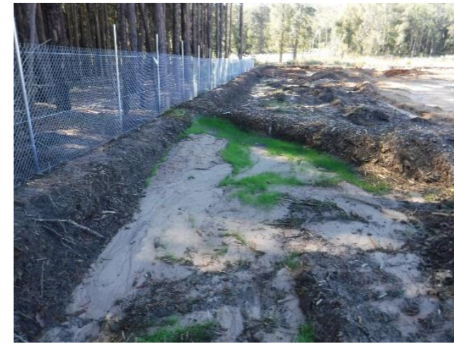
Example photo of a compacted mulch berm on steeper grade with an upslope facing groyne
